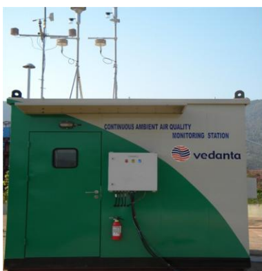
Continuous Ambient Air Quality Monitoring Station
