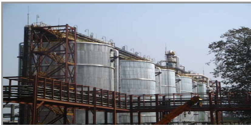
Pre – desilication area
