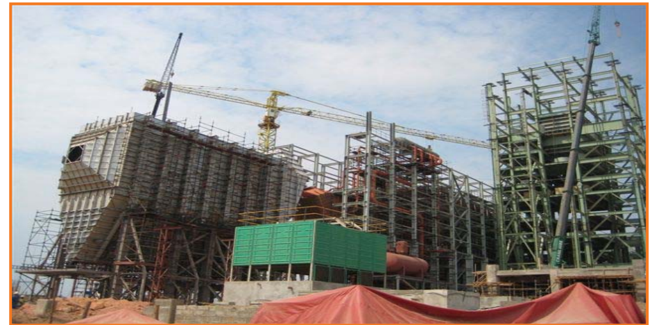
View of ESP, Boiler, Smelter building
